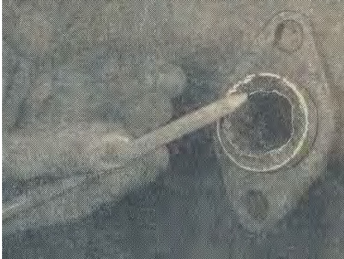
Left: Figure 3. Badly carbon-clogged exhaust pipe illustrates how the heat valve can get stuck with carbon. This condition is hard to detect without disassembling. It may be suspected when the car loses its normal top speed, and especially if overheating persists. Replacing clogged pipes with new ones is the only cure, and is helpful in correcting mysterious cases of vapour lock.
